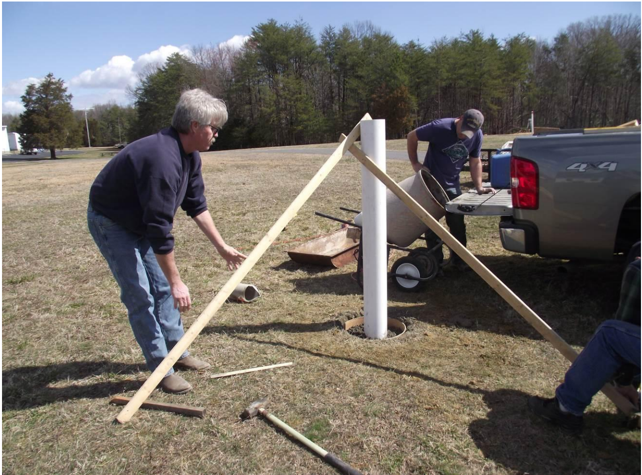
Figure 9. Level the top and brace the PVC pipe. With the PVC pipe positioned at the desired location in the hole, attach one end of a 2- by 4-inch board to the top of the PVC pipe using 2-inch drywall screws. Attach the other end of the board to a wooden stake driven securely into the ground using 3-inch drywall screws. Repeat this process using a second board at a 90 degree angle. Double-check the position and level of the PVC pipe in the hole to be sure it is securely braced.
