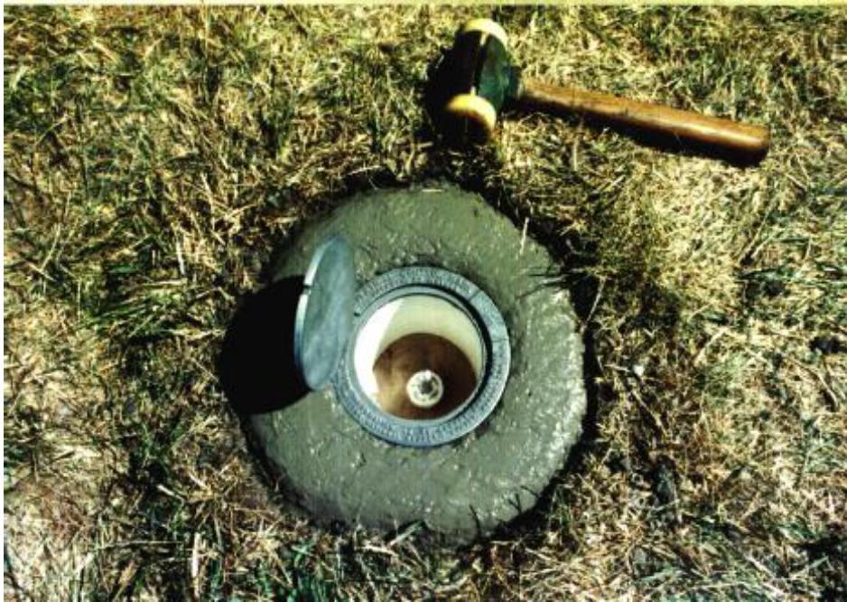
Finished Monumet, Cap Open Note: Very Neat Appearance, SS Rod Centered in PVC, PVC Centered in Concrete, Concrete Round (Not “Mushroom” Shaped), No Concrete on Logo Cap, No Concrete on the Ground
