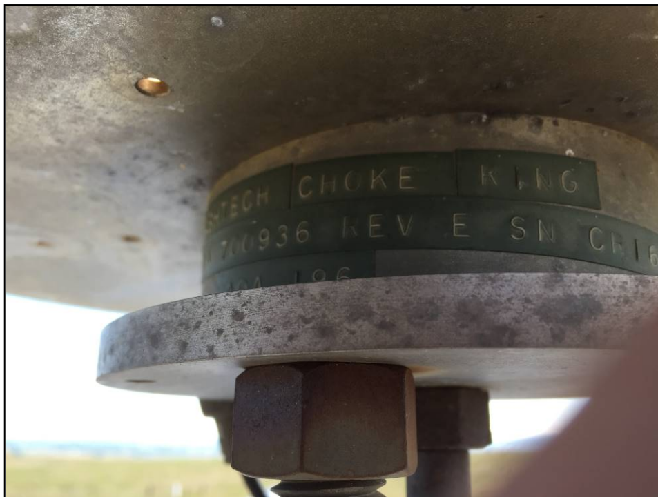
TMGO atop steel tower
