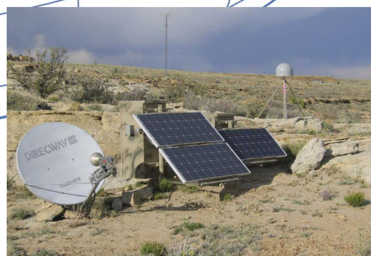
Figure 2. CORS site P028 (owned/operated by UNAVCO, www.unavco.org ); CORS such as this help define the geometric component of today's NAD83 and the new geometric datum.
